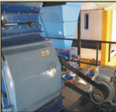
HAMMER MILL (20 TPH)
